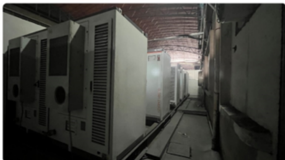
Zhejiang 2.4MWh C&I Energy Storage Power Station
