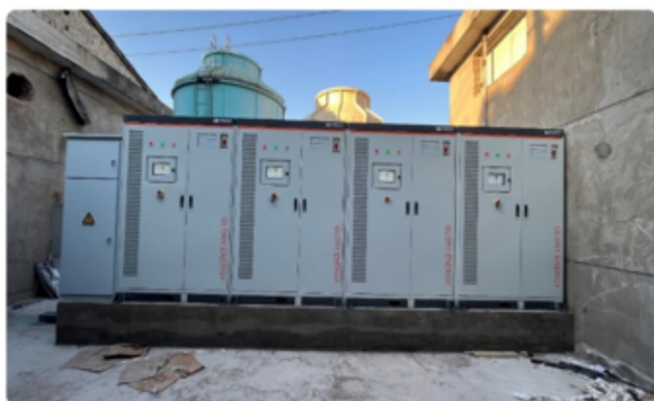
Zhejiang 860kWh C&I Energy Storage Project
