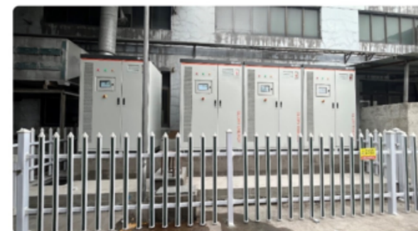
Zhejiang 800kWh C&I Energy Storage Project
