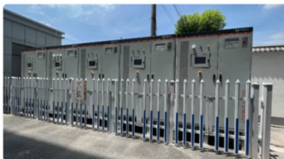
Zhejiang Jinhua 1MWh Renewable Energy Storage
