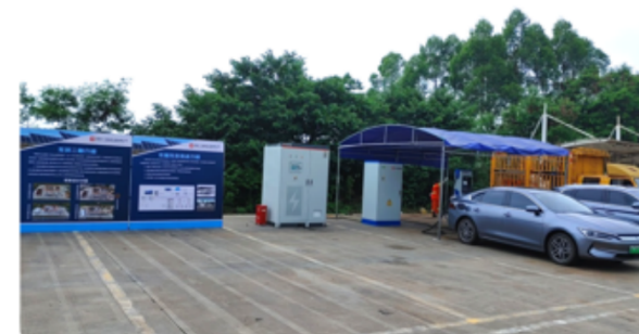
Shenzhen 215kWh Integrated System
