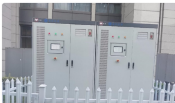
Zhejiang Hangzhou 400kWh Energy Storage Project
